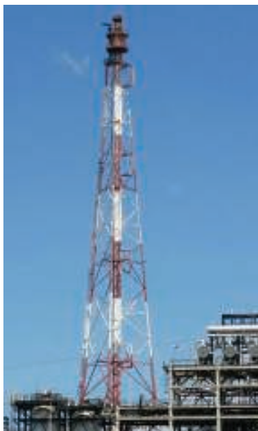
FIGURE 8. The ability to eliminate air ingress through proper engineering design and ongoing maintenance and troubleshooting is an important factor in optimizing the reliability and safety of flare systems
