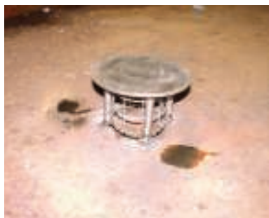
FIGURE 6. The new design of the drain cap with legs (based on bird-cage wire mesh) prevents direct plugging due to refractory or unburned coke debris
