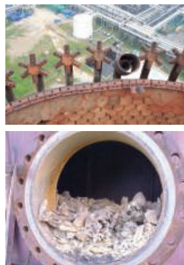
FIGURE 5. The castable refractory shown here is partially heat damaged and has become loose at the inside of the flare tip (top). The excessive build-up of refractory debris and unburned coke amounted to about half of the height of the 24-in.-dia. manhole (bottom)
