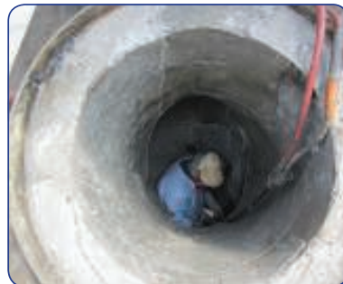
A Diamond Refractory specialist works on the flue gas inlet of an FCCU
